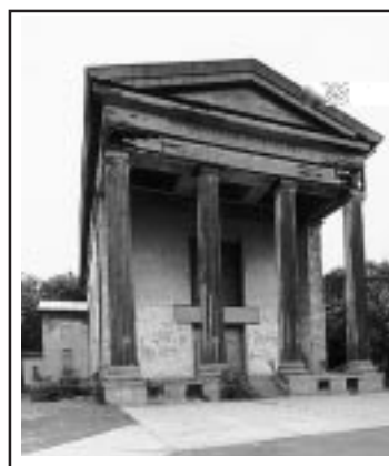
The Dutch Reformed Church's structural system has been stabilized with the help of local, state and federal funds, and a community group is exploring reuse opportunities. Photograph by Michael Gabor
